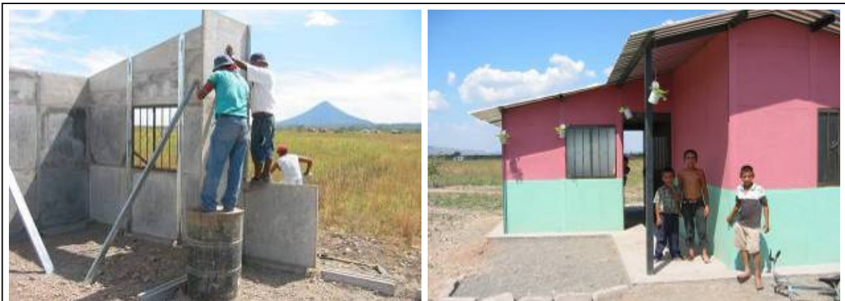
Construction of houses at La Palmerita – after waiting for six years in black plastic shelters, 112 houses were built in less than three months. Living conditions have dramatically improved but much more needs to be done for this to become a self-sufficient, thriving community.
